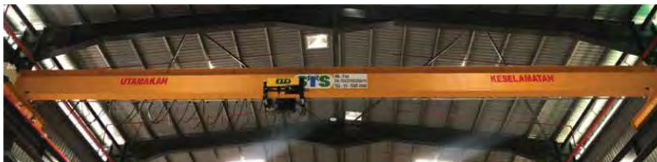
5 Tonne Single Girder Overhead Travelling Crane.
