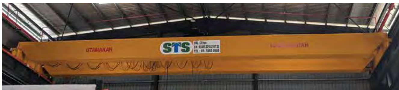
20 Tonne Double Girder Overhead Travelling Crane.
